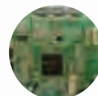
3 DC inverter control
