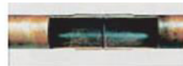
Nitrogen blow not performed (Oxidation scale)
