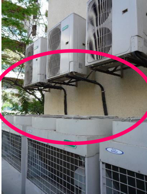
Short circuit of discharge air flow
