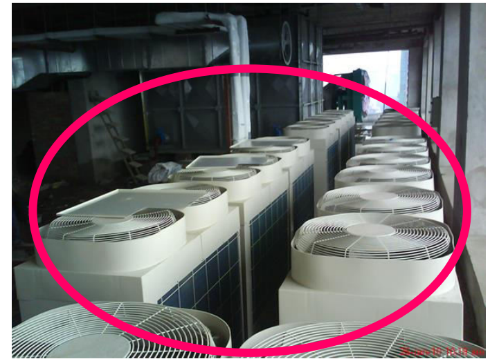
Short circuit of discharge air flow
