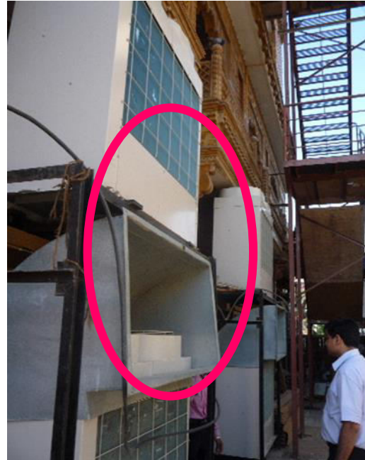
Short circuit of discharge air flow
